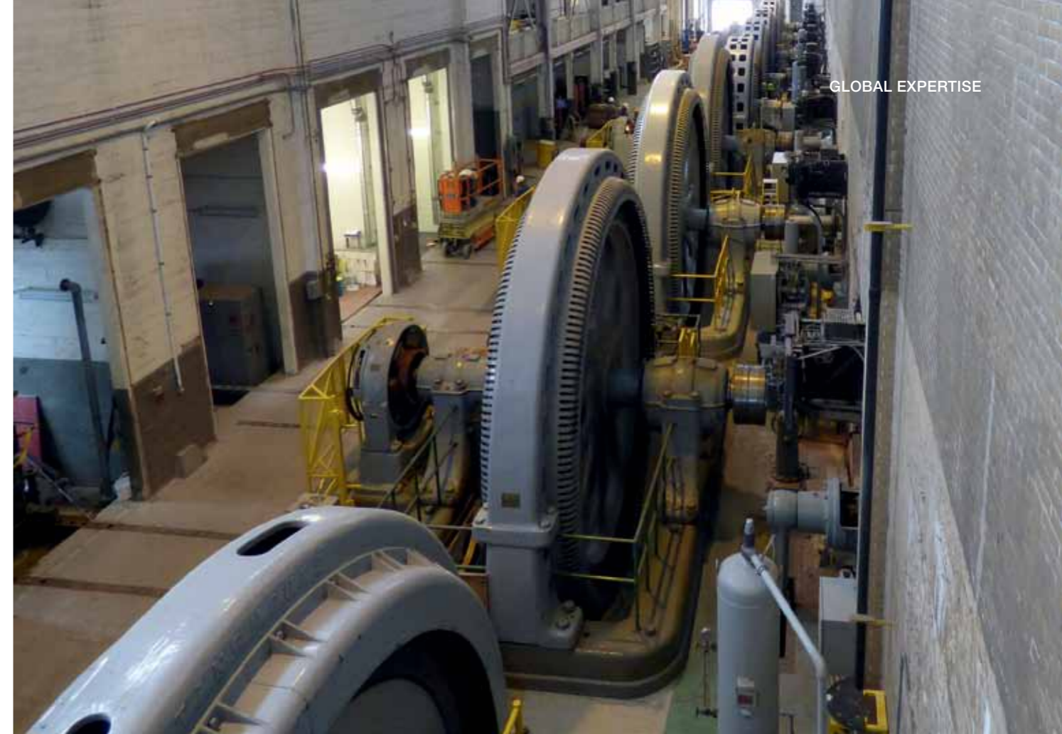
Improved original: Voith-restored 1920s components at Pointe du Bois.
