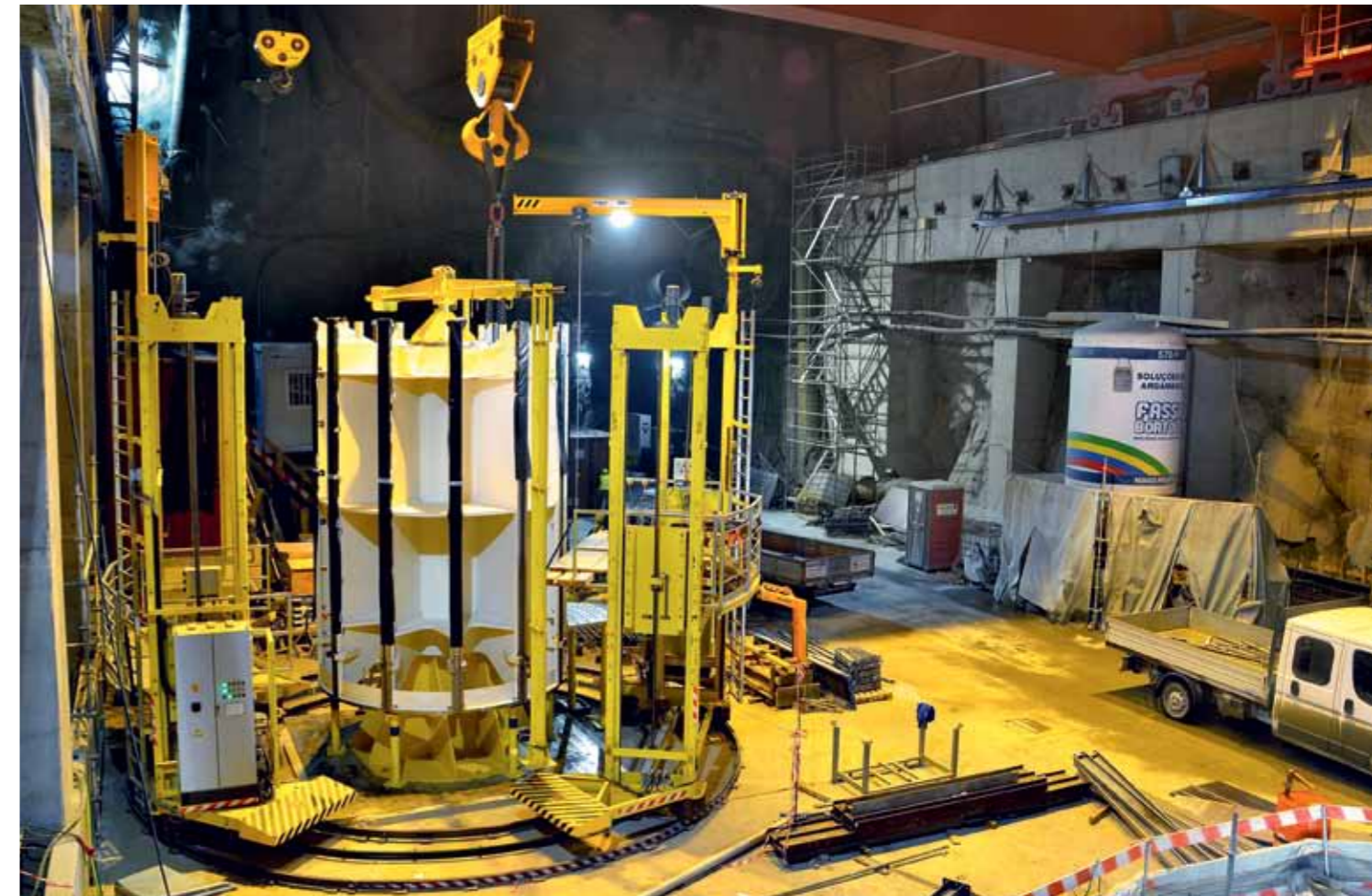
The rotor hub with the newly developed, semi-automatic stacking platform at the pre-assembly spot, shortly before lamination bundling starts.
