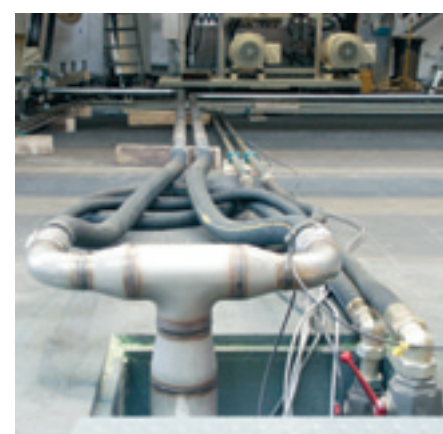
Fig. 2: Hydraulic unit supply piping to the Janus MK 2 from the Nipco roll test rig.
