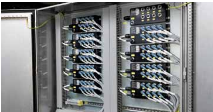
Separate, protected installation of the electrical units.
