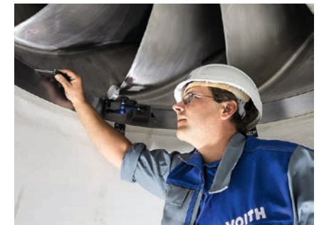
A Voith engineer inspects a turbine on site at Reisseck II.
