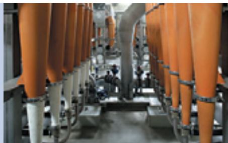
EcoMizer cleaner plant.
